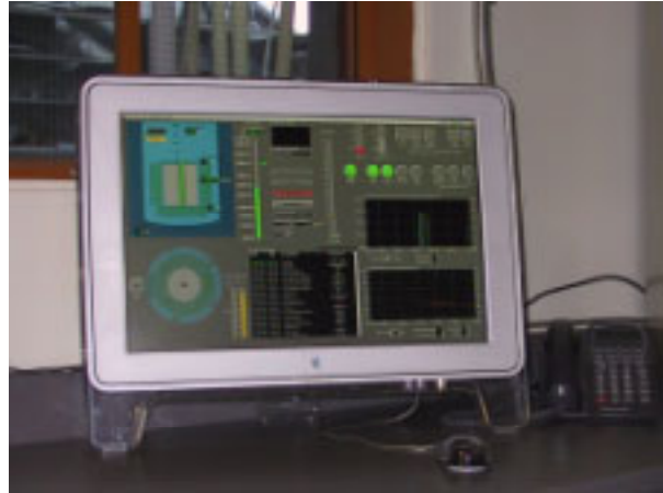
Figure 2 - SIRCIS Operator Workstation
