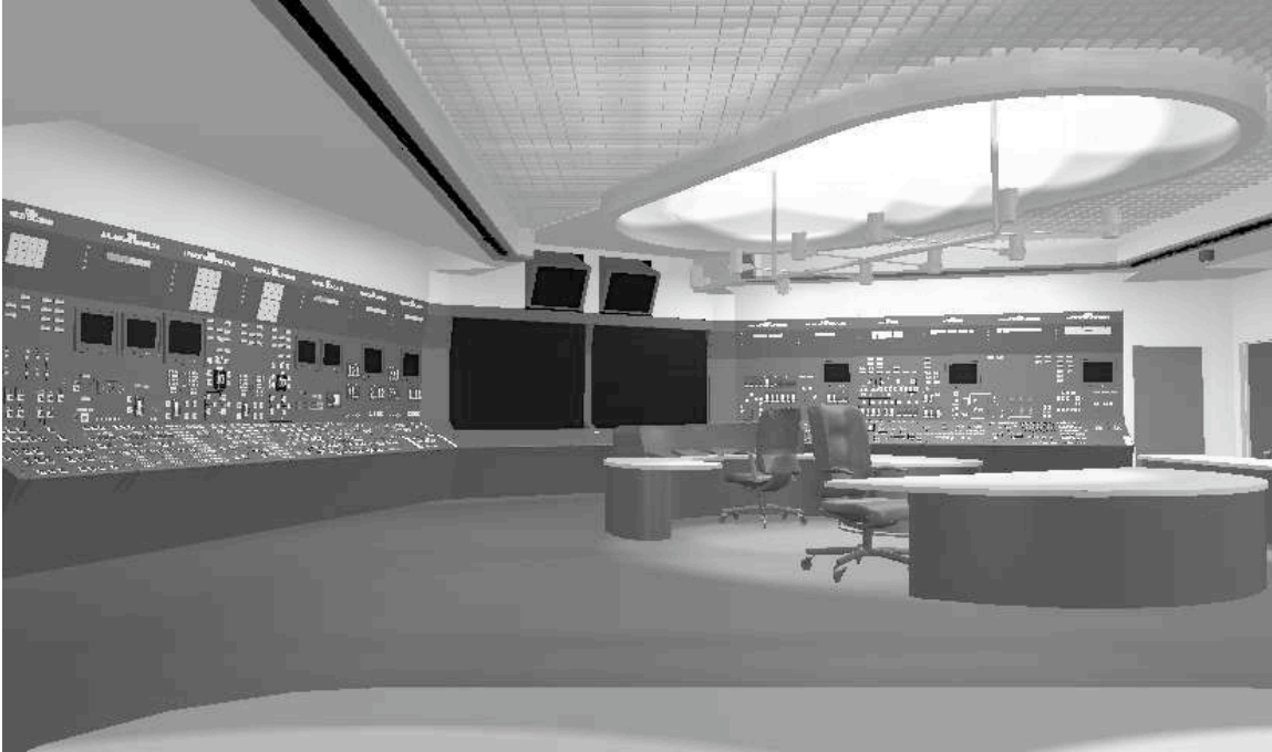
Figure 3 QCNP CANDU 6 Control Centre Preliminary Draft
